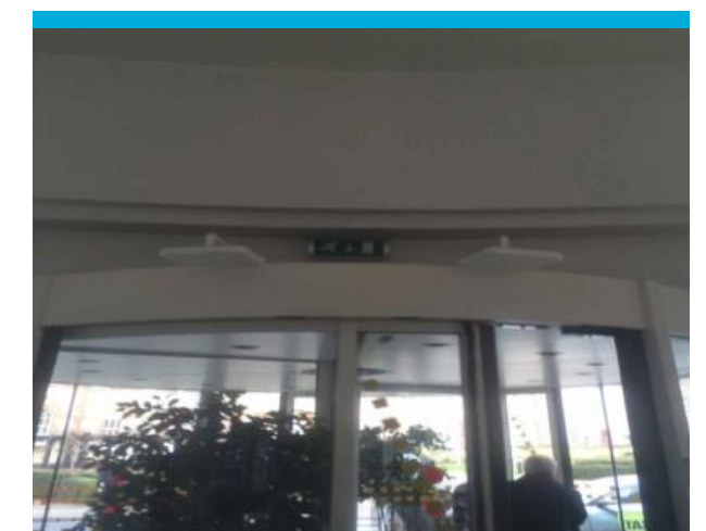
Figure 4: RFID readers installed at doors in the hospital.
